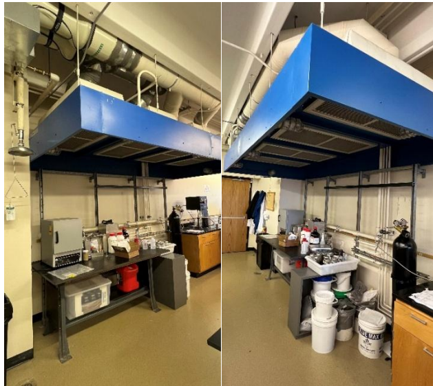
Figure 1—The left and right view of the outdated canopy ventilation exhaust in EN 4042, alongside ovens, retorts, high-temperature equipment, flammable chemicals, oil-based samples, and nanoparticles.
